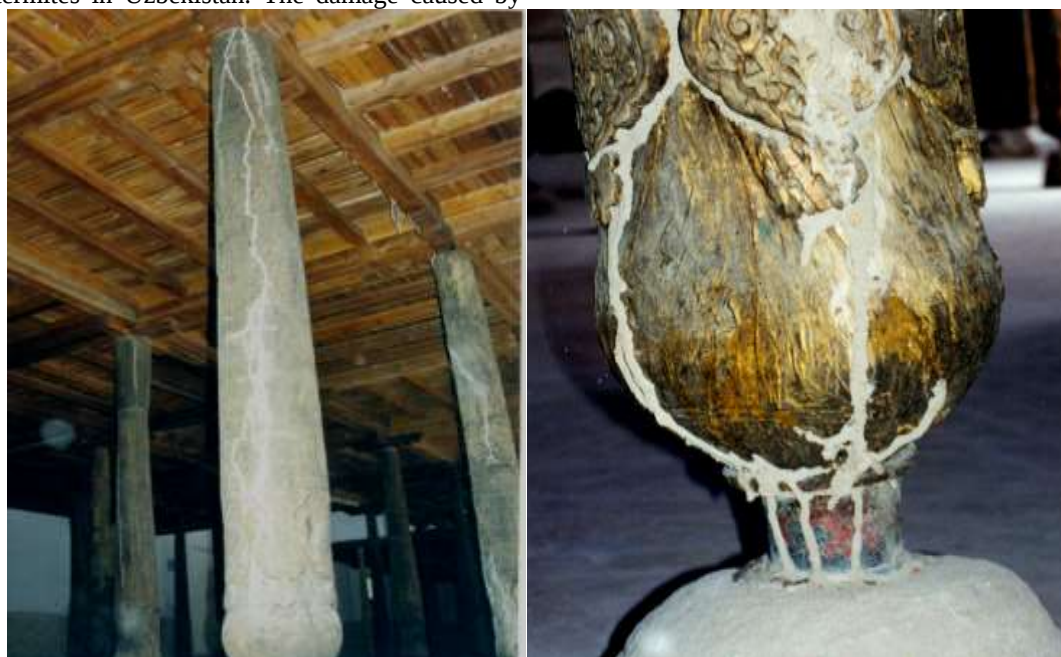
Picture 1 The damage of termites to the wood structures of the mosque "Juma" in the historical complex of Ichan-Kal'a, Khiva, Uzbekistan.
