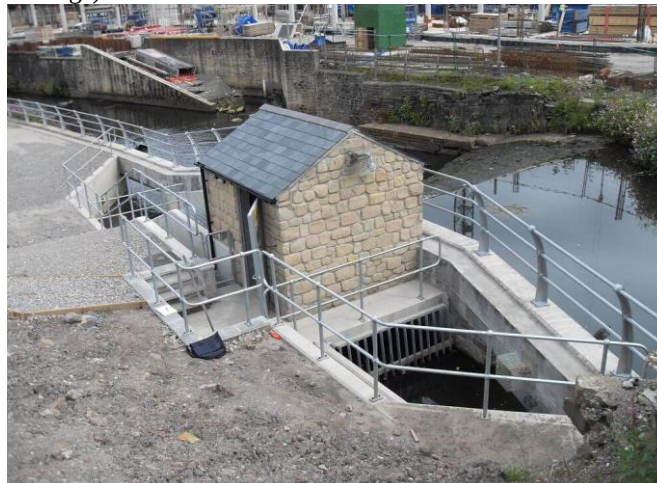
Figure 6. The turbine house at the Rochdale hydropower scheme [25]
